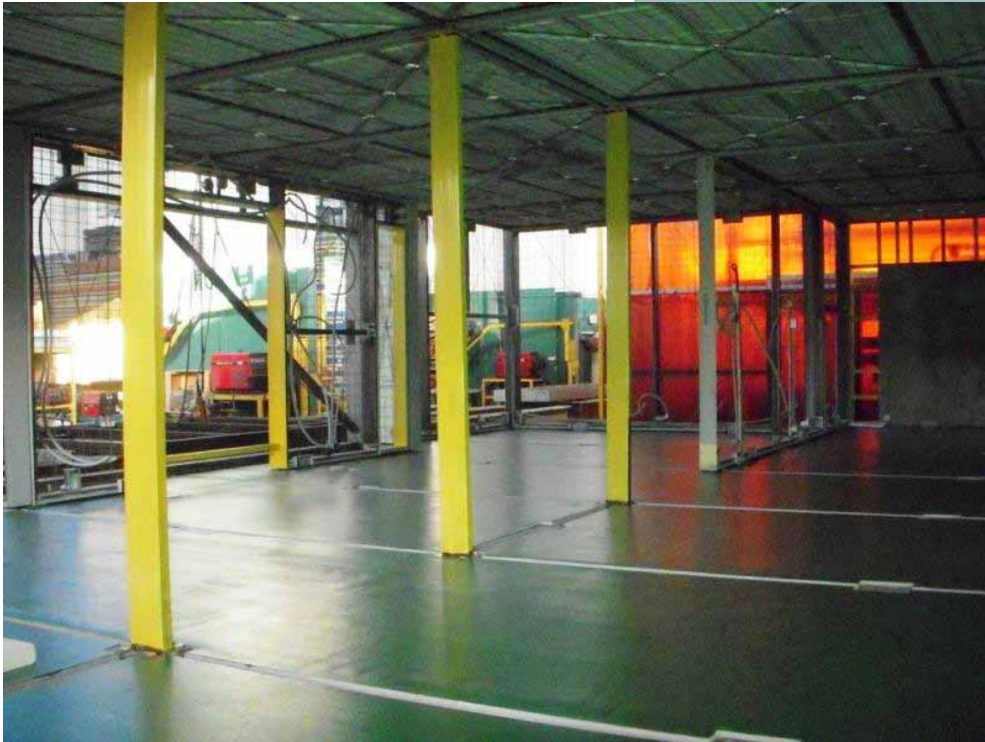
INTERNAL VIEW OF PRESENTATION CENTER OFFICE SPACE SHOWING THE PERFECTLY SMOOTH FLOOR PANELS SEALED IN GREEN. THE 3 YELLOW VERTICAL SUPPORTS ( SHOWN ABOVE ) ARE TEMPORARY AND WILL BE REMOVED ONCE THE PANEL FRAME DRY RUN ASSEMBLY IS DISMANTLED FOR CONCRETING THE PANELS.
