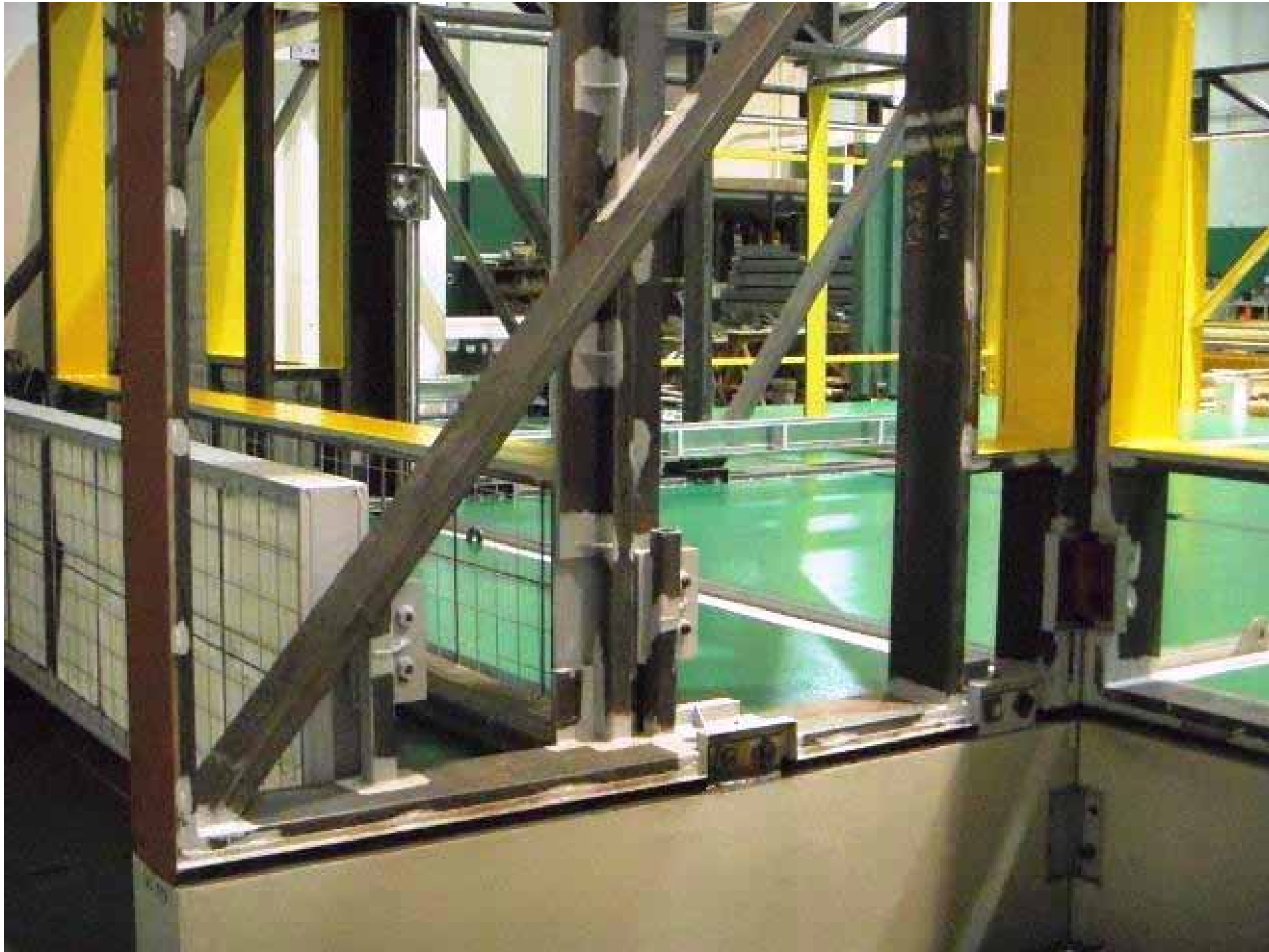
THIS PICTURE SHOWS AGAIN THE CONNECTIONS BETWEEN THE EXTERIOR IHI WALL PANELS AND THE IHI FOUNDATION BEAMS AS WELL AS VARIOUS OTHER CONNECTIONS BETWEEN THE PANELS
